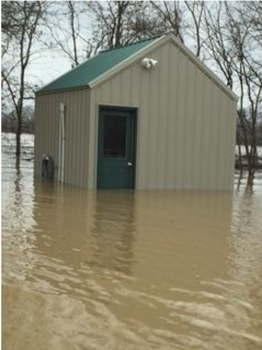
Figure A-15. Flooded Equipment Building
